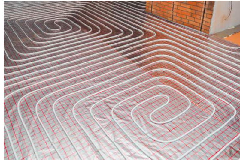
FLOOR HEATING ALL ROOMS
